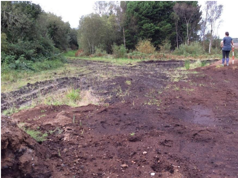
Plate 95: Proposed Grid Connection Route in bog margin before connecting into proposed substation site.
