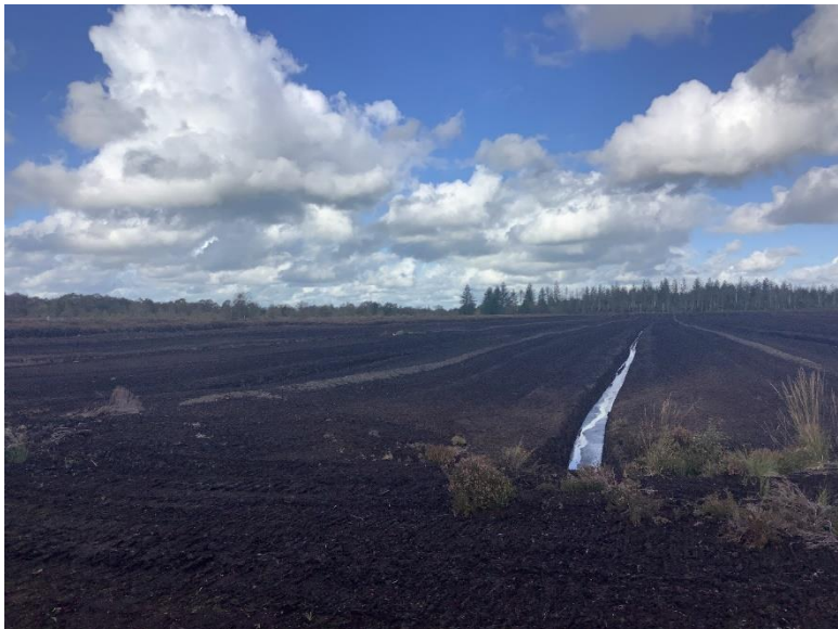
Plate 3: General view of T1 and associated hardstand (2020), looking NW.
