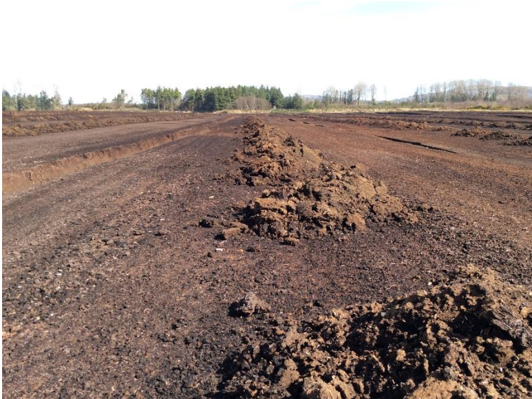
Plate 23: Hardstand and general view of proposed access track to T6 (2017), looking NE.
