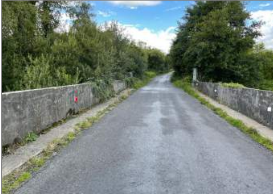
Figure 2 View along Clonava Bridge, showing the grass growing along the road in front of the concrete verges
